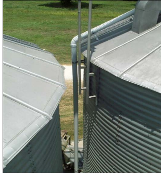
Permanent recirculation tubing
