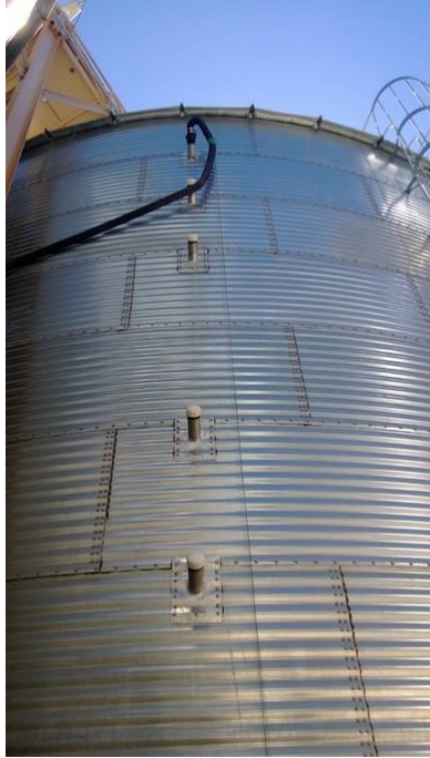
Temporary recirculation tubing
