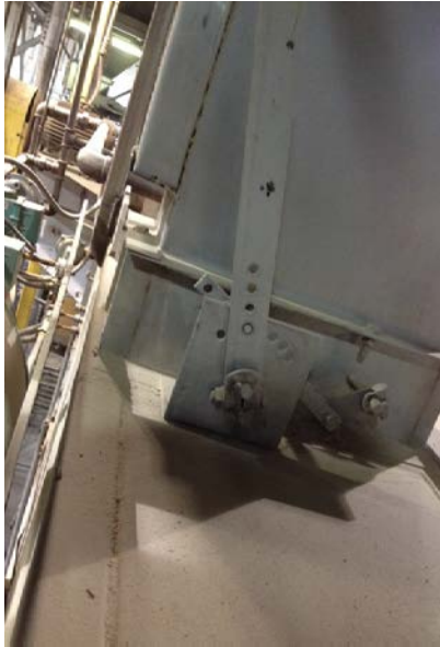
Burner damper setting
